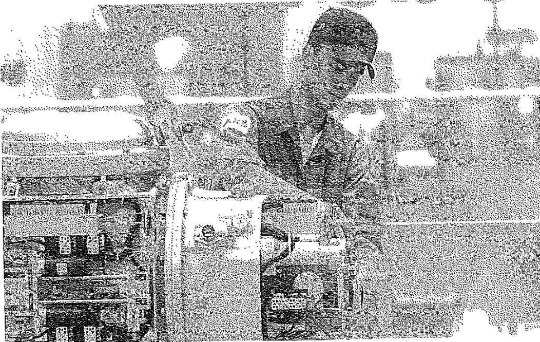
Mechanical routine test of the make-proof earthing switch
